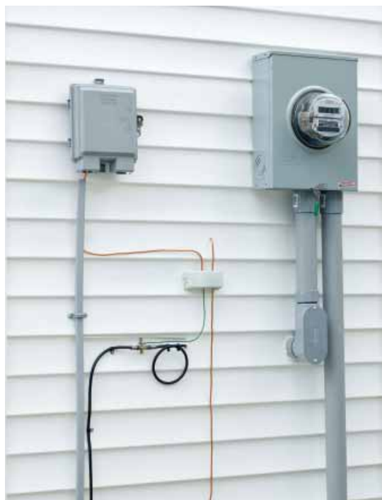
Intersystem Bonding Termination - Typical installation bonding the electrical system to the telephone and CATV systems.
